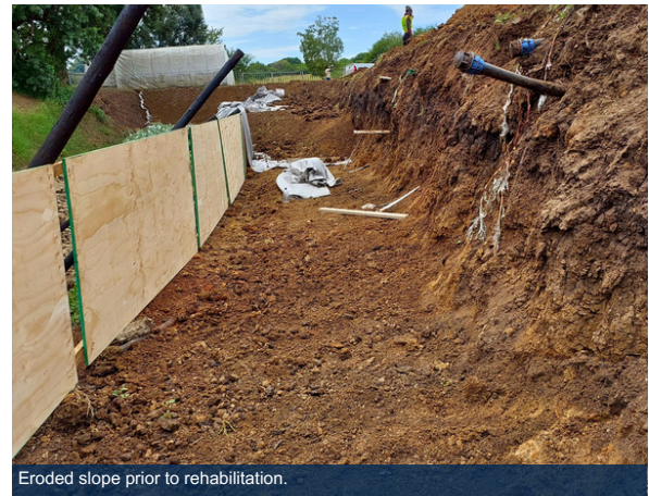
Eroded slope prior to rehabilitation.
